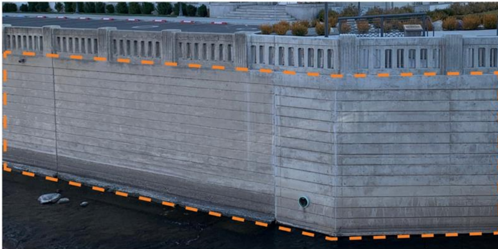
Flood Wall Texture North Side- Repeated at Virginia Street Bridge Near Post Office
